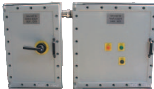
160 kW star-delta motor starter protected by MCB
